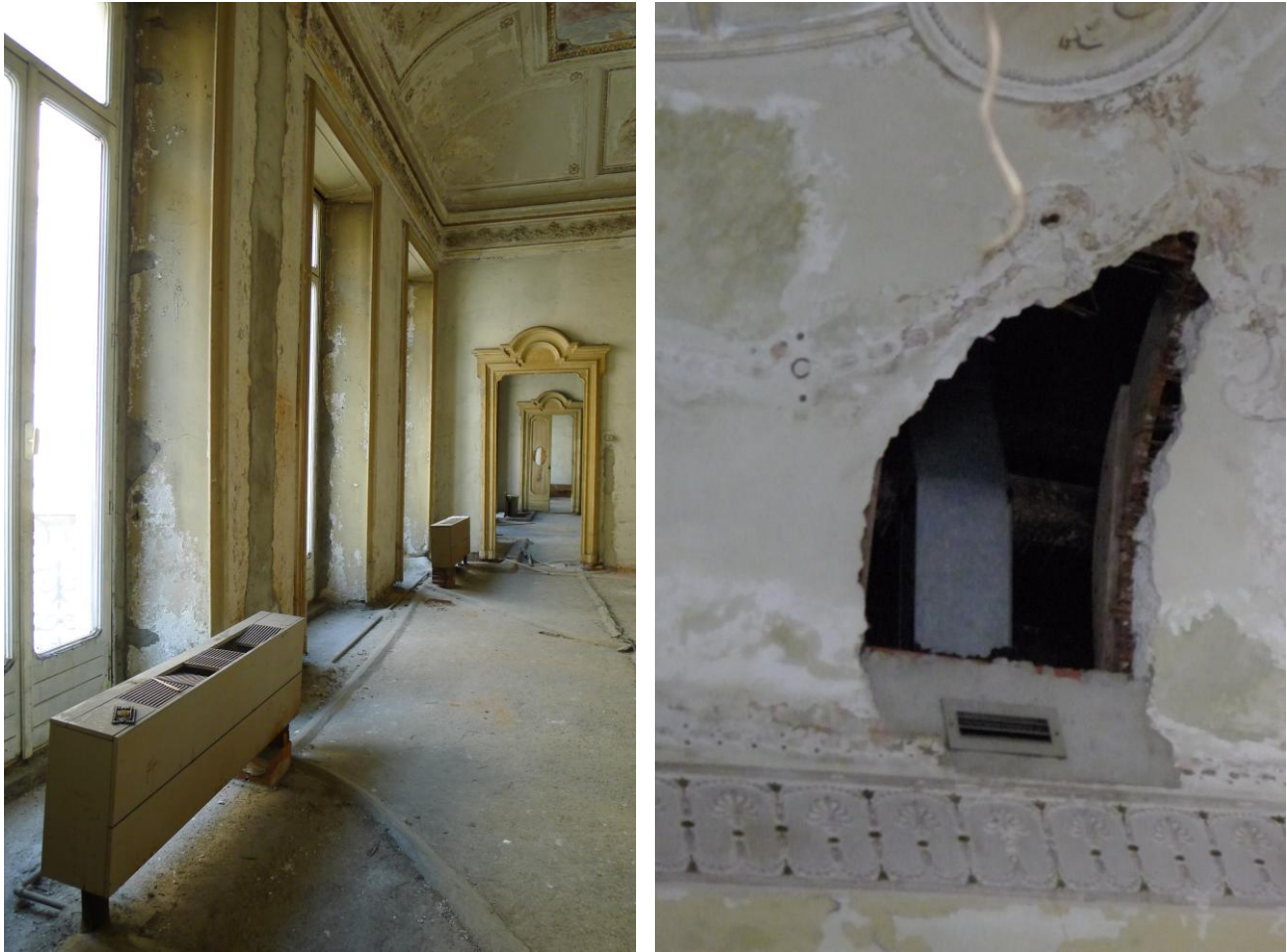
Fig. 0.1 – Example of a very invasive introduction of modern climate control devices within a historic building (Pictures by C. Manfredi).
